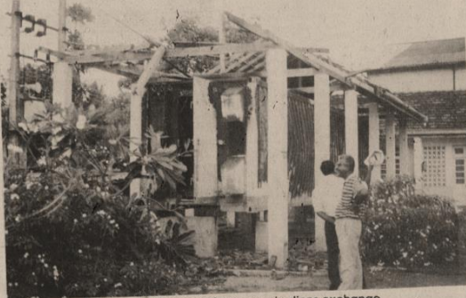
Destroyed Kalmunai telecommunications exchange
